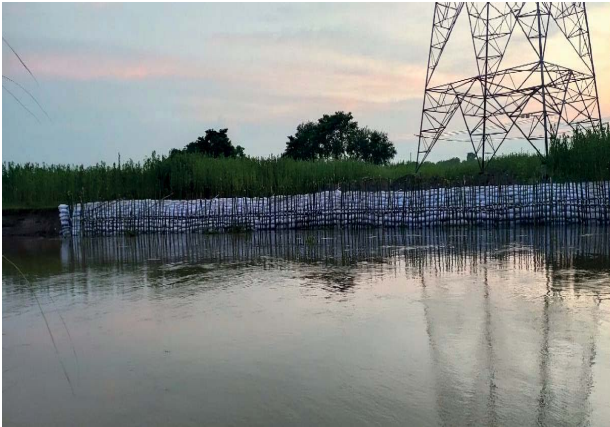
After- Photographs of Tower no. 97 (Tower protection by using Bamboo piling & Geo Bags)
