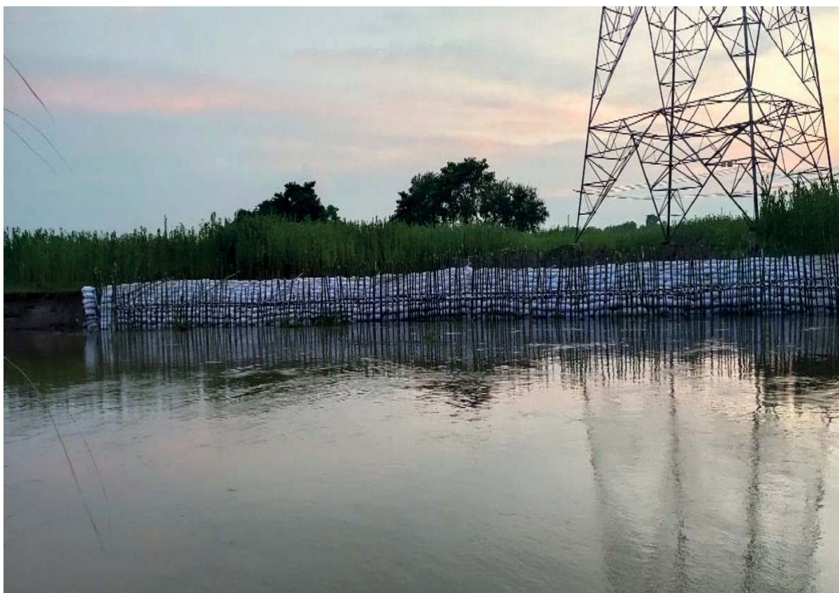
After- Photographs of Tower no. 97 (Tower protection by using Bamboo piling & Geo Bags)
